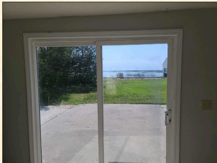
Sliding door screen is missing.
