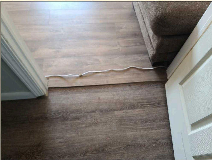
Open seams/partially finished flooring observed.
