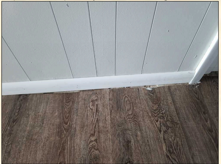
Bedrooms Floor Condition
