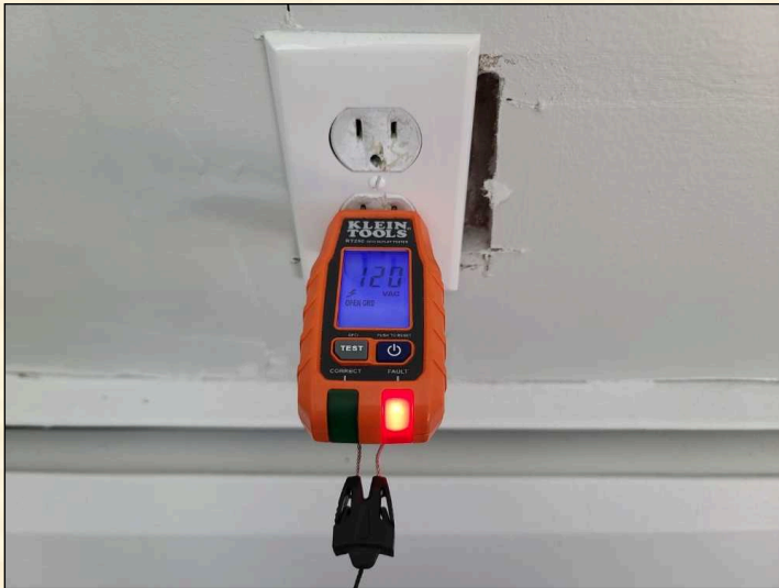
Open ground (or 2-wire) outlets present. This means that the 3rd (round) part of an appliance plug is not getting ground protection.
