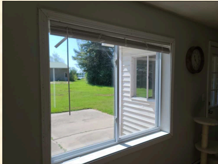
Missing screens observed.
