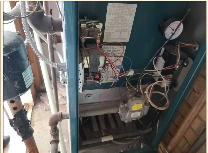
Heat/AC Heater Condition
