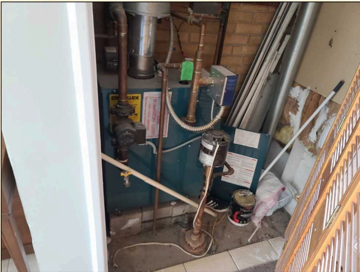
Heat/AC Heater Condition
