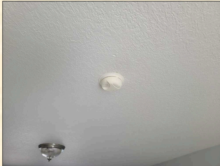
The smoke alarm(s) did not operate when tested.
