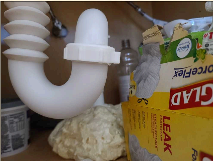
Sink drain assembly is loose. Leaks observed.
