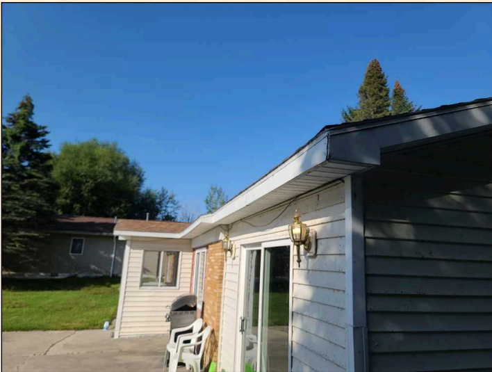
Partial gutters - Full installation recommended to keep water away from structure. Water can weaken the foundation and deteriorate the siding. Be sure to install splashblocks or extensions to carry water away, and keep water from areas such as driveways or walks where it can be an ice hazard in winter.
