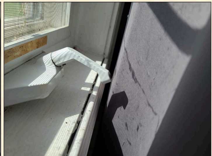
Missing hardware at the kitchen windows. Repair as needed.
