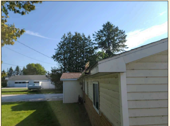
Downspouts missing and/ or broken; recommend installation.
