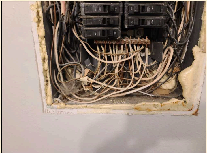
Electrical Electrical Panel
