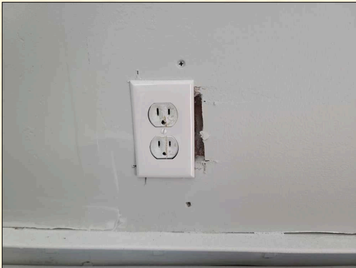
Gap around Outlet observed.
