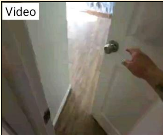
SW bedroom (2&3) doors bind in the jam.
