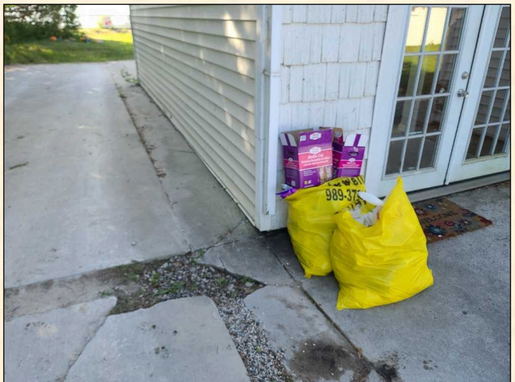
Downspouts missing and/ or broken; recommend installation.
