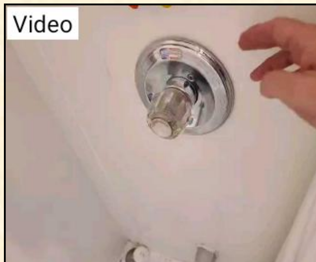
Loose escutcheon plates noted. These should be refastened and caulked to keep water from infiltrating the walls.
