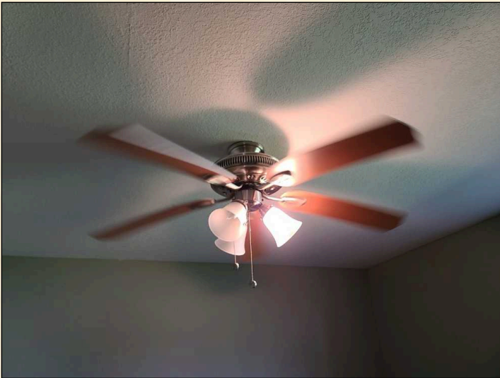
Operated normally when tested, at time of inspection.
