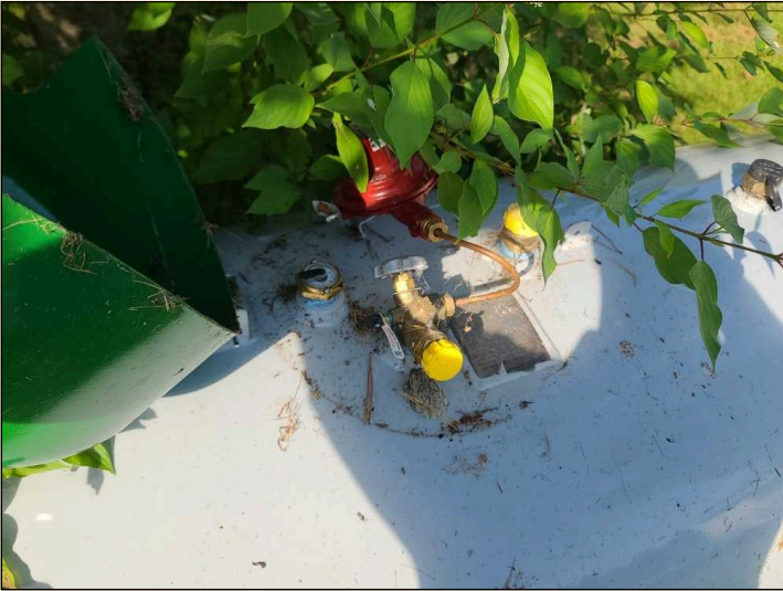
Grounds Main Gas Valve Condition
