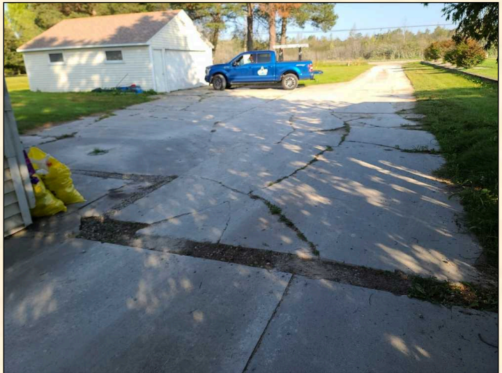
There are numerous areas of damaged concrete surfaces. Concrete replacement is expensive. Recommend a concrete specialist provide an estimate for repair and or replacing.
