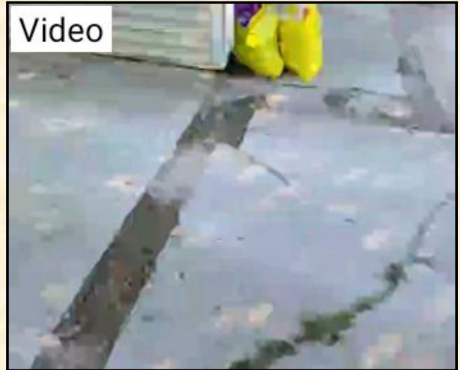
Video Uneven slabs at the driveway. This is a potential tripping hazard. Recommend repair and or replacement of the displaced walks.
