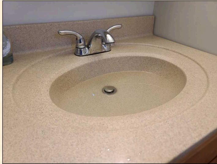
Slow drain at sink. Recommend clearing.
