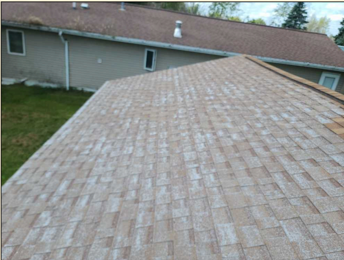
Serviceability of roof is questionable; it should be evaluated and repaired as necessary by a professional roofing contractor.
