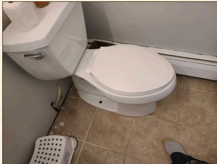
Toilet loose and may need re-anchoring.
