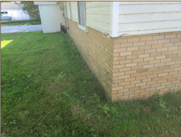
Downspouts missing and/ or broken; recommend installation.
