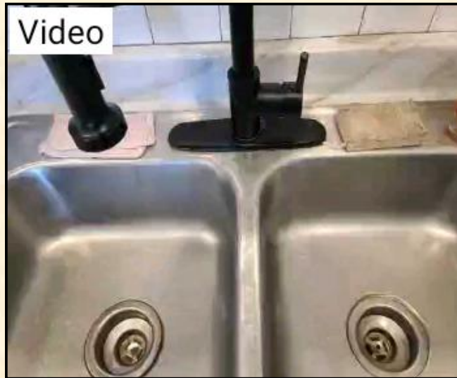
Faucet is loose, suggest securing as necessary.
