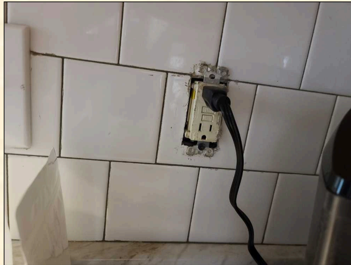
Outlet cover(s) missing.
