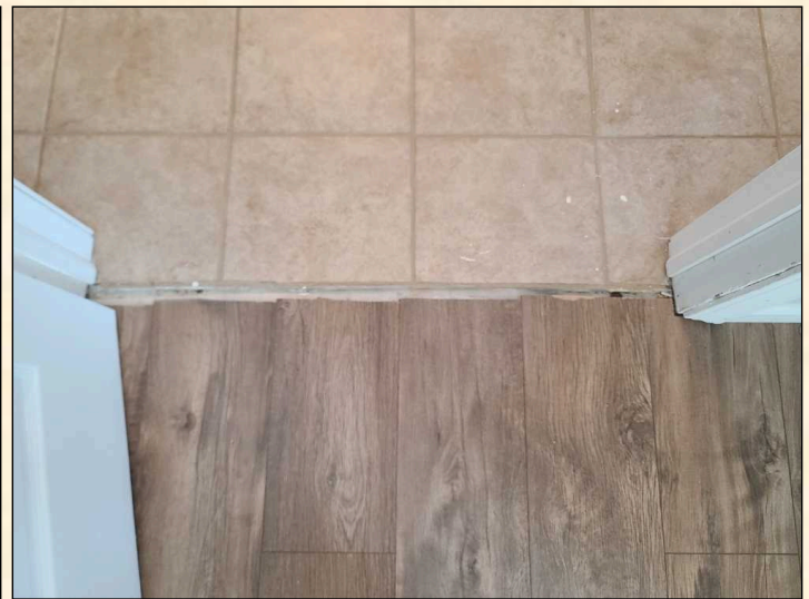
Open seams/partially finished flooring observed.
