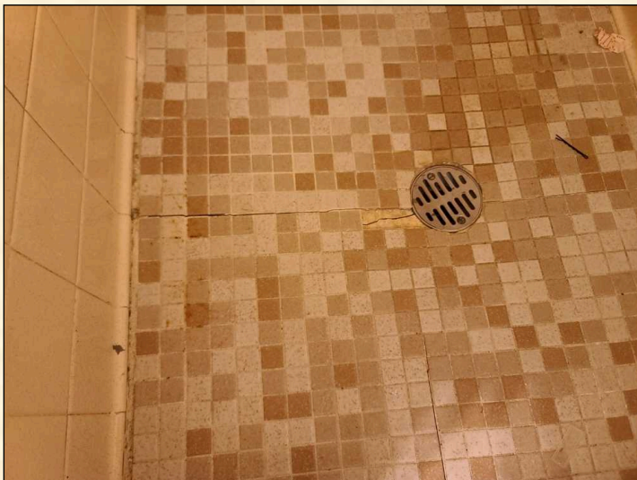
Tile base is cracked.
