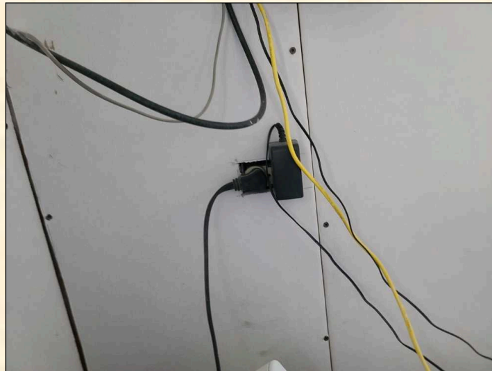
The laundry receptacle should be GFCI protected type.
