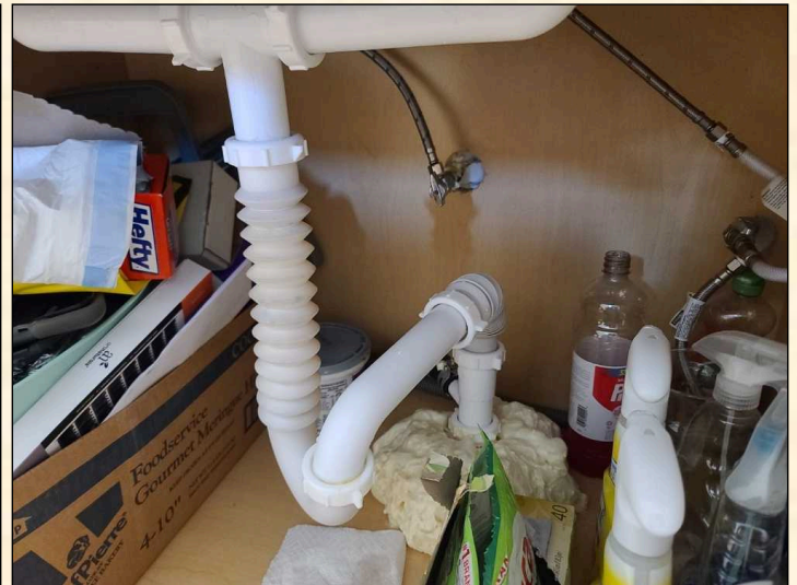
Flex drain observed, these are subject to frequent clogging.
