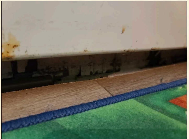
Open seams/partially finished flooring observed.
