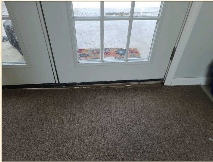
Moisture damage around the door trim
