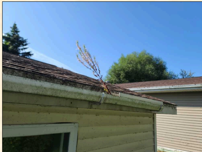
Clean gutters: Significant amounts of debris evident.
