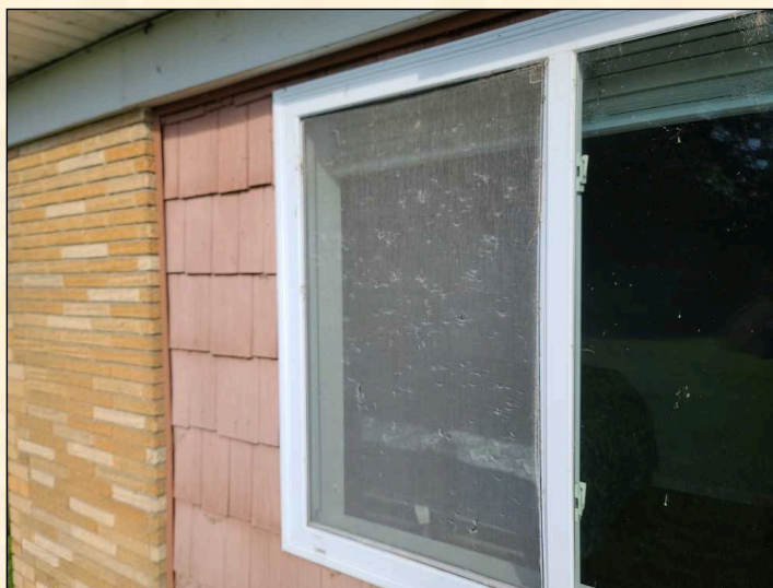
Some window screens damaged.
