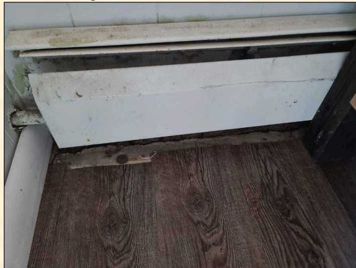
Open seams/partially finished flooring observed.
