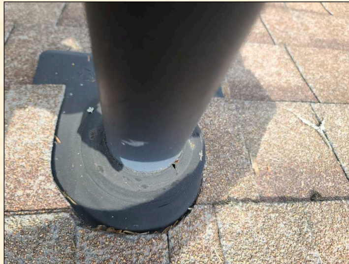
One vent boot needs to be resealed or replaced.
