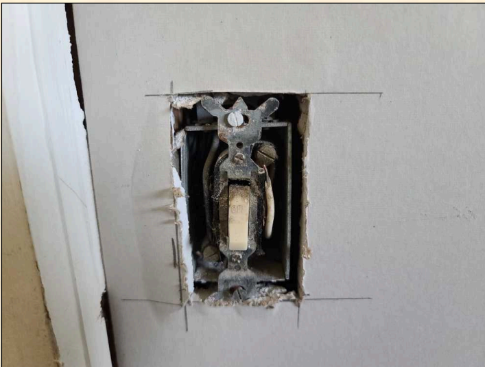
Switch cover plates missing.
