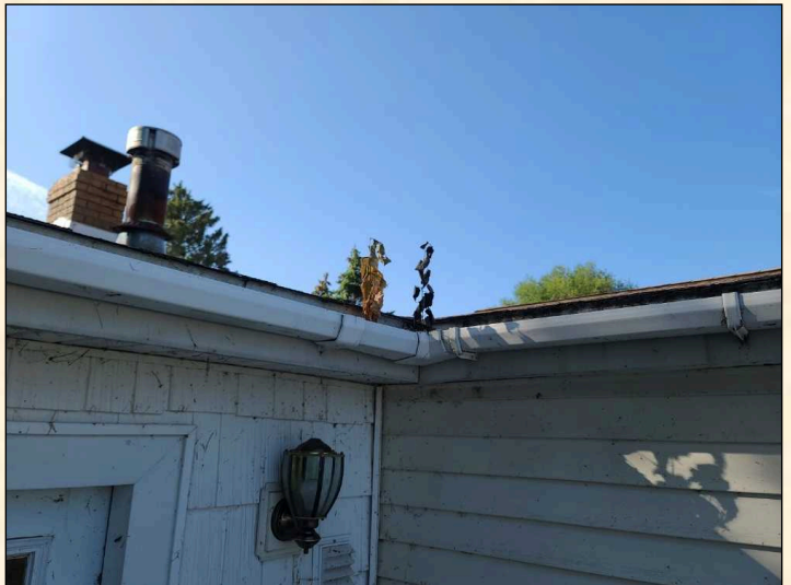
Clean gutters: Significant amounts of debris evident.
