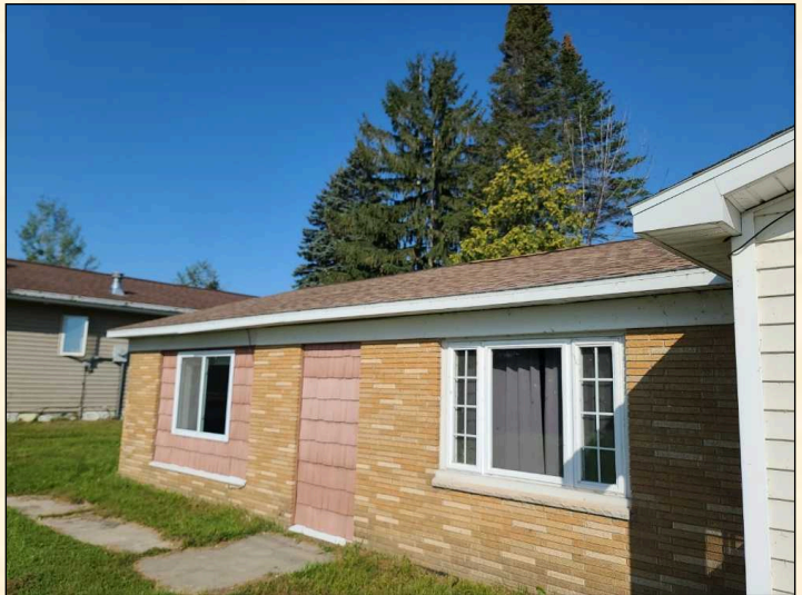
Partial gutters - Full installation recommended to keep water away from structure. Water can weaken the foundation and deteriorate the siding. Be sure to install splashblocks or extensions to carry water away, and keep water from areas such as driveways or walks where it can be an ice hazard in winter.
