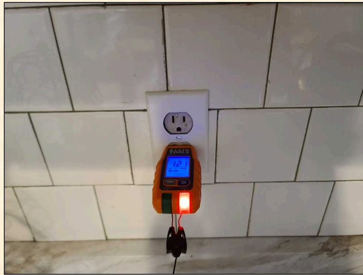
Non GFCI receptacle noted at the countertop.
