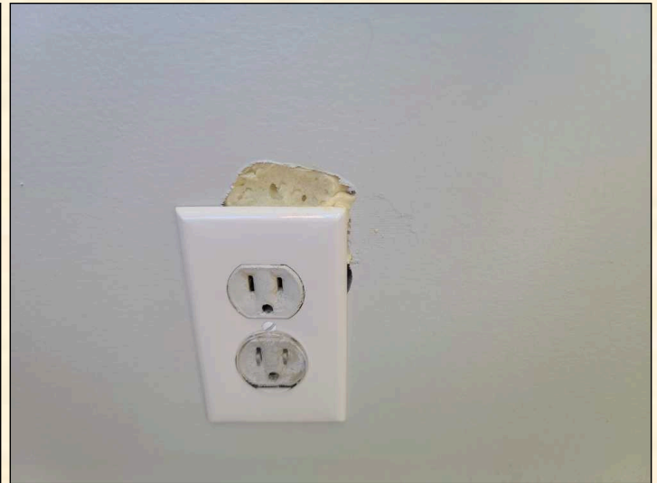
Gap around Outlet observed.
