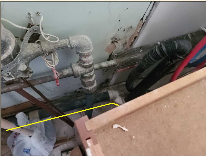
Drain pipe should be a minimum of 6 " off the floor.
