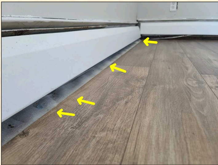
Open seams/partially finished flooring observed.
